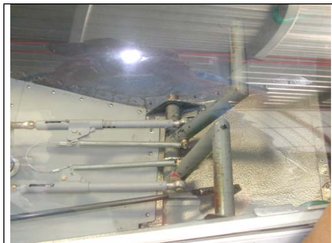
With the gust locks installed a disengaged ruddervator caused pedals to be offset.
